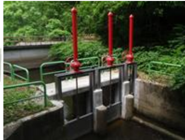
Water gate cylinder
